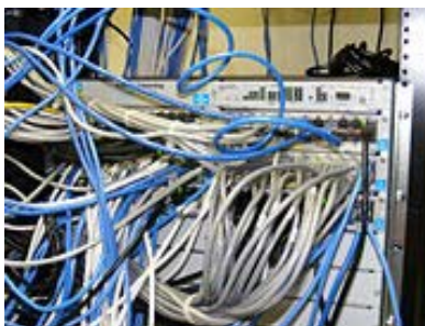
A rack-mounted switch with network cables
