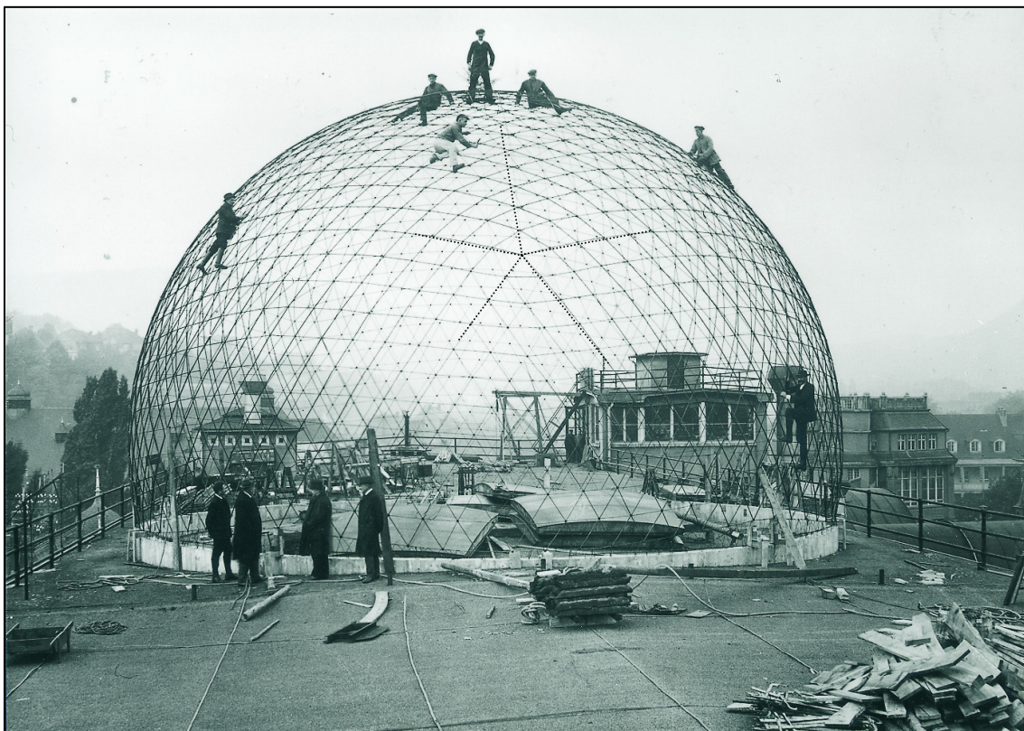
Figure 2.6: Image during the construction process of the dome that is going to be studied in this chapter. We can clearly appreciate the icosahedrons inspired pattern of the mesh.
