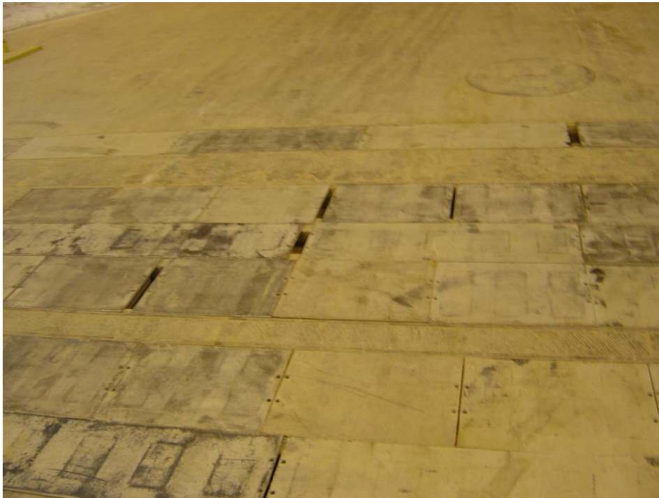
Figure 11.2. Uneven part of the floor of the LHC tunnel at point 6
