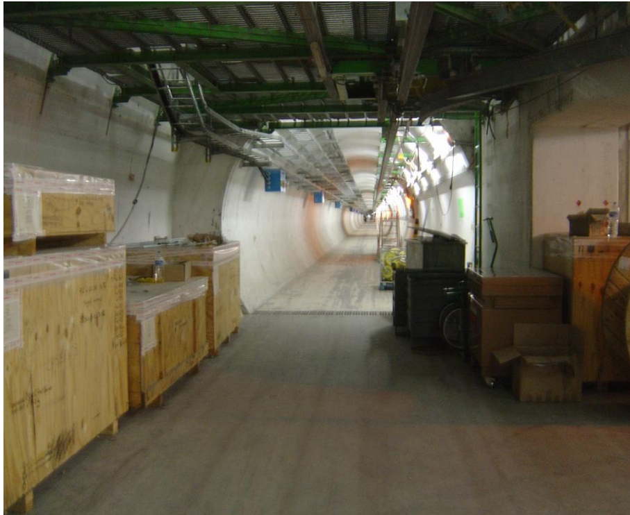
Figure 11.1. View of a section of the LHC tunnel at point 6
