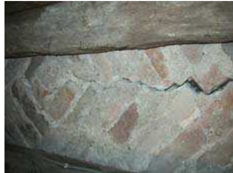
Figure 3.35: Cracks in the vaults
