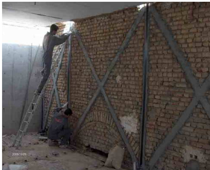
Figure 3.12: Shear strengthening by CFRP plates in one side at Shariati museum in Tehran, Iran in November 2005. (Motavalli M, 2005)
