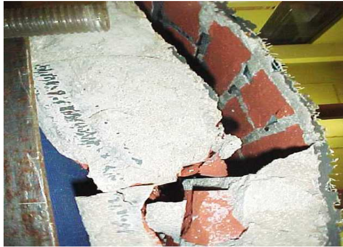
Figure 3.4. Combined failure mode of brick- compression failure and laminate cohesive failure (Ayman, 2007).
