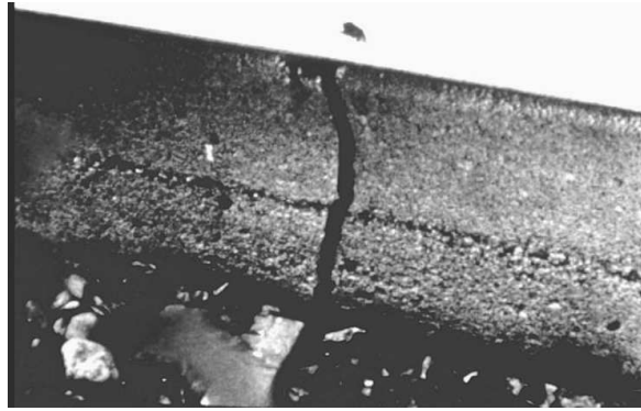
Figure 2.24: Crack in Masonry Foundation (California seismic society, 2005)
