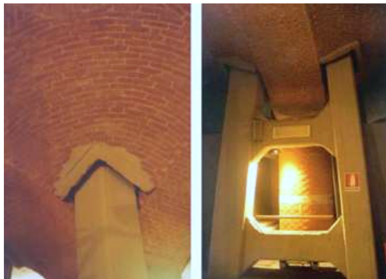
Figure 2.9: R.C. structure substituting the original one in the "Mole Antonelliana", Turin, Italy. (EU-India cross program, 2006)
