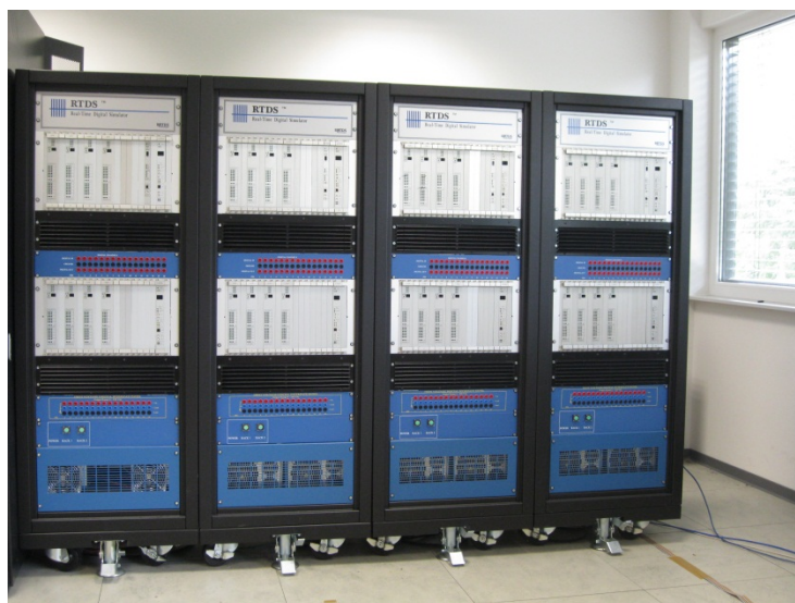
Fig. 6.1 RTDS hardware at E.ON ACS Institute
