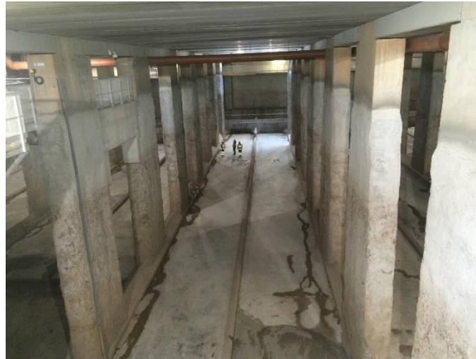
Figure 13. La Estrella retention tank. First visit.
