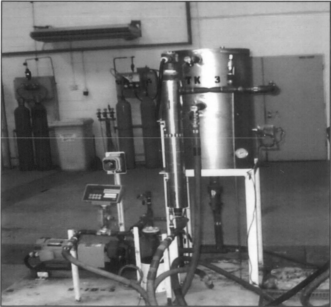
Figure 3.13: Photograph of the Heating System
