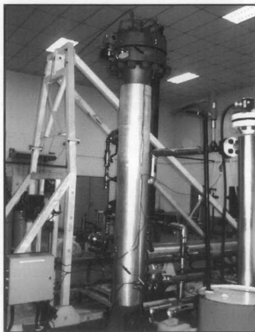
Figure 1.3: Photograph of the oil tank storage
