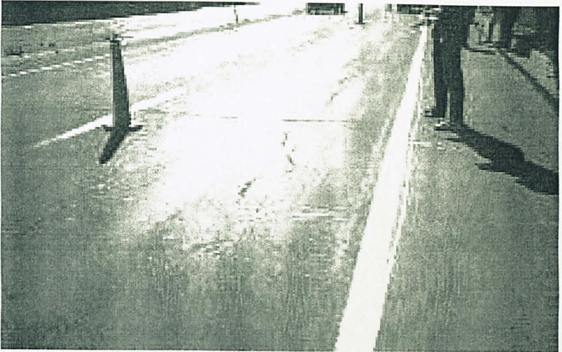
Figure 2.7 Low Severity (Source: FHWA, 2003)
