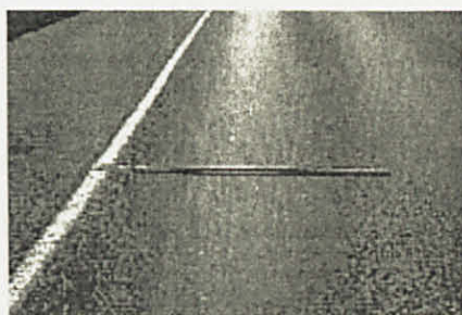
Figure 2.3 Rutting (Source: FHWA, 2003)
