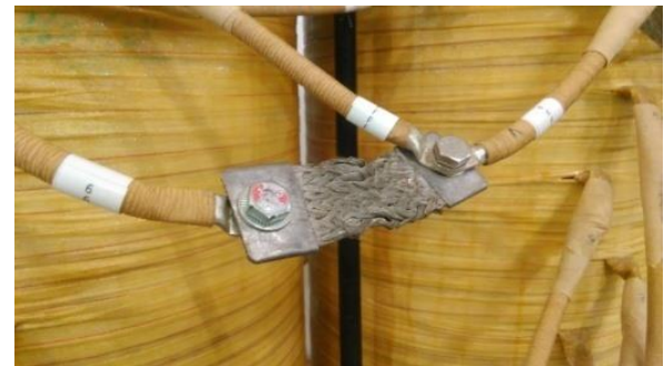
Fig. 6. Turn-to-turn short circuit
