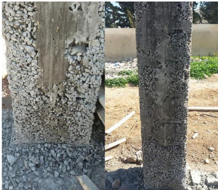
Figure 9.15 An example of concrete works failure
