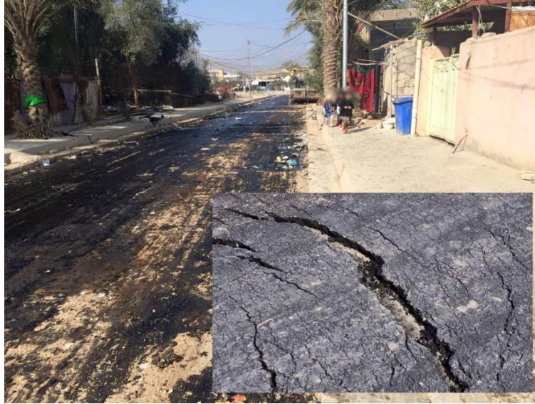
Figure 9.14 A sample of asphalt pavement failure
