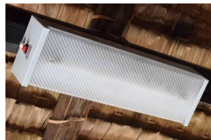
Figure 13. LED Emergency Light
