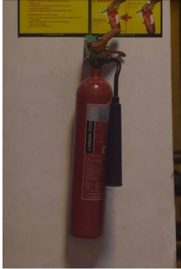
Figure 10. CO 2 fire extinguishers
