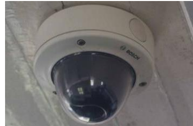
Figure 12. CCTV camera (right)
