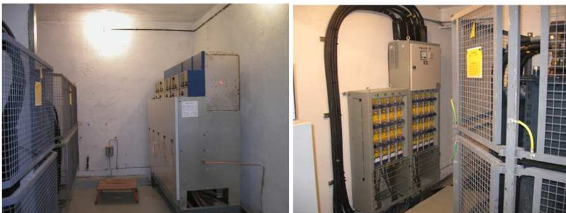
Figure 25: “Processing Centers” Source: Iberdrola Distribution
