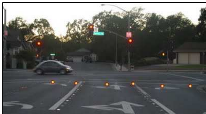
Figura 2–34: Light Guard System instalado.
