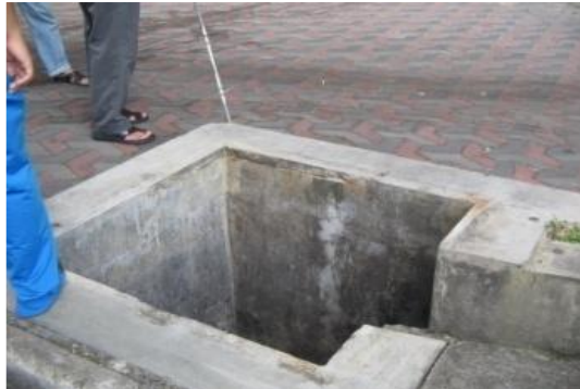
Figure 5.5: The uncovered manhole can bring danger situation to the users especially people with visual impaired.
