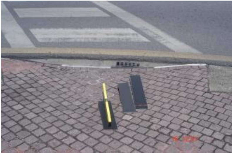
Figure 6.12: Uneven curb cuts at pedestrian crossing
