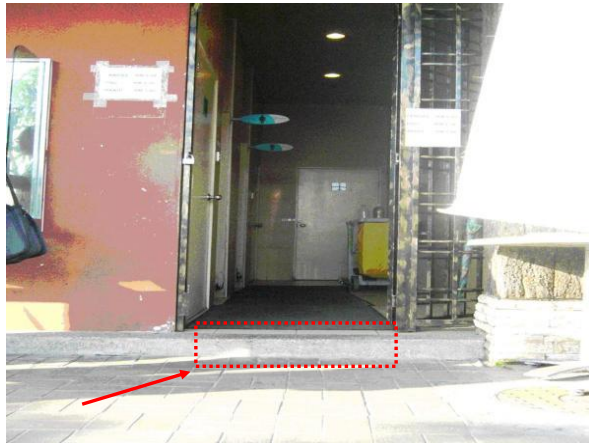
Figure 6.6: Inappropriate drop for entrance to toilet at the Festive Street Mall
