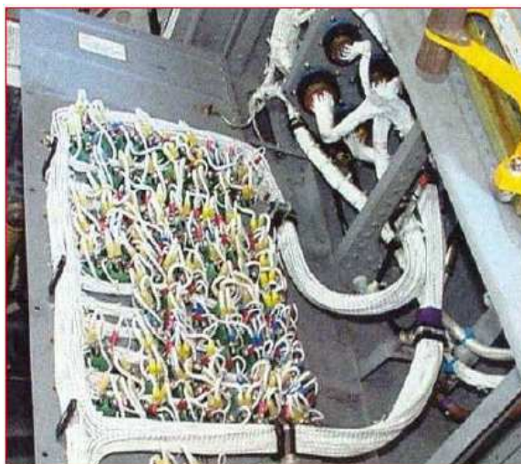
Figura 45. Panel de Circuit Breaker
