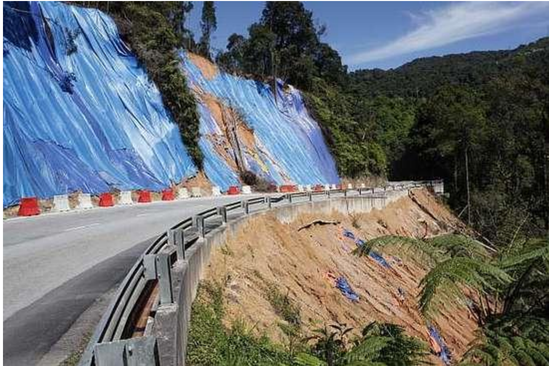
Construction of road needs to blend the existing terrain to avoid landslide.
