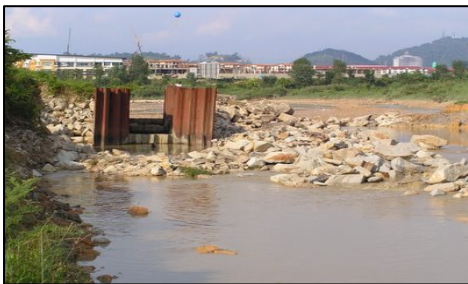
Fig. 8. Broken bund on the site
