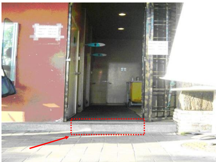
Figure 6: Inappropriate drop for entrance to toilet at the Festive Street Mall
