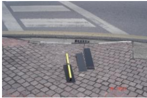
Figure 12: Uneven curb cuts at pedestrian crossing
