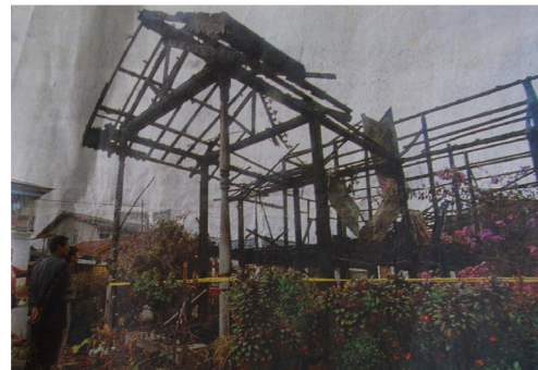
Figure 2: The wooden building of Rumah Pak Ali that built on 1876 was destroyed by fire on 20 Oct. 2003.
