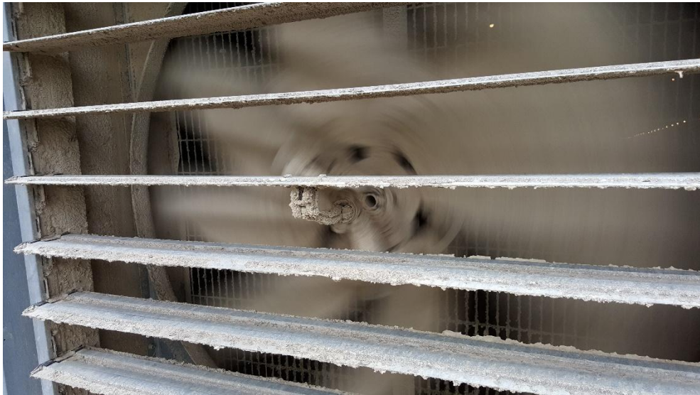
Fig. 20 Dust accumulated on blades and shutters of target tunnel fan
