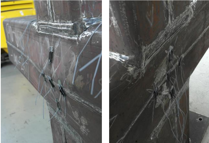
Figure 3.16 The chord sidewall buckled inward and outward (X90-650-1.000-26.7)
