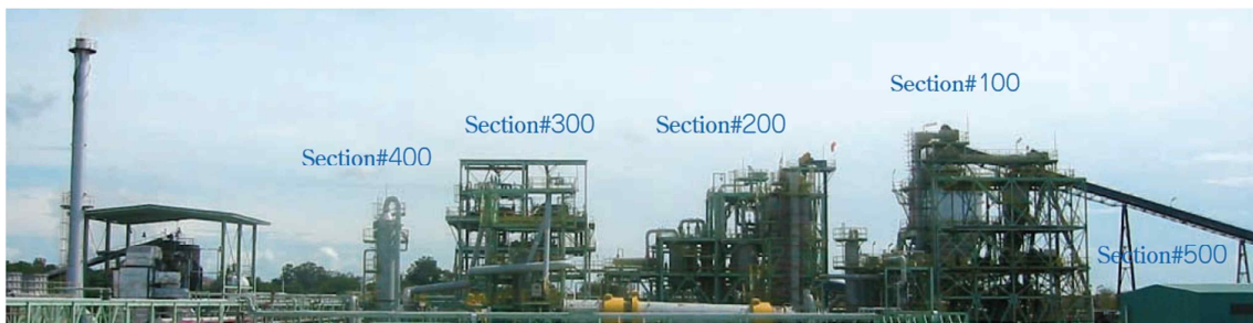
Fig 3-10 Photo of UBC Plant
