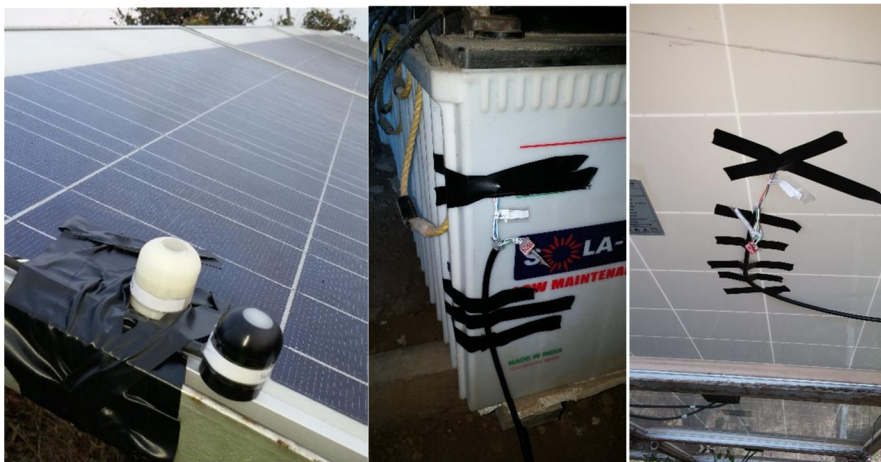
Figure 93. Images of sensor installation in Thingan, Nepal
