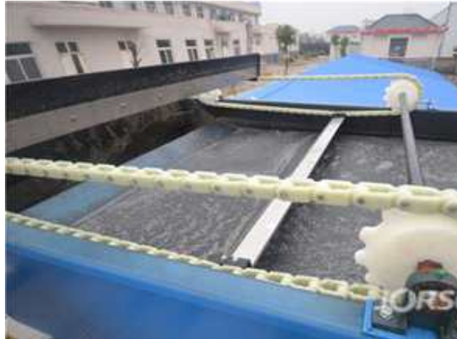
Fig. 2.6 Chain - flight removal system
