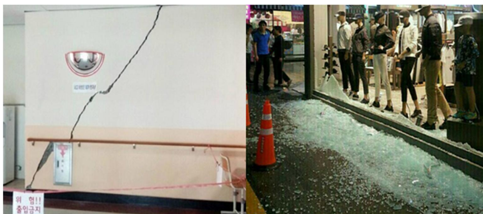
Fig. 1-1 Damages of the earthquake in Gyeongju
