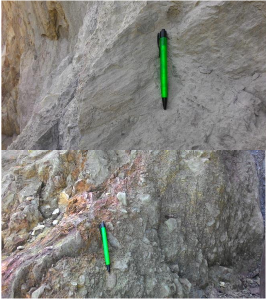
Fig 5. Fault breccias and slickenside feature indicating the slope was affected by a fault system.
