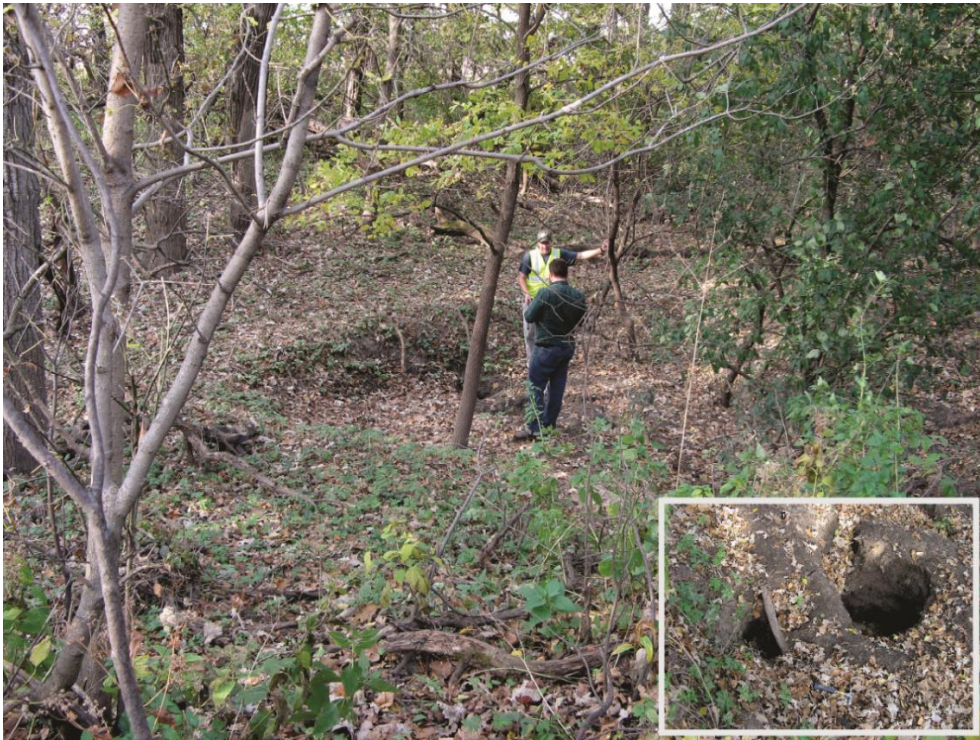
Fig. 2: A developing sinkhole found in the mapping area. The lower-right picture shows the central hole of the structure.
