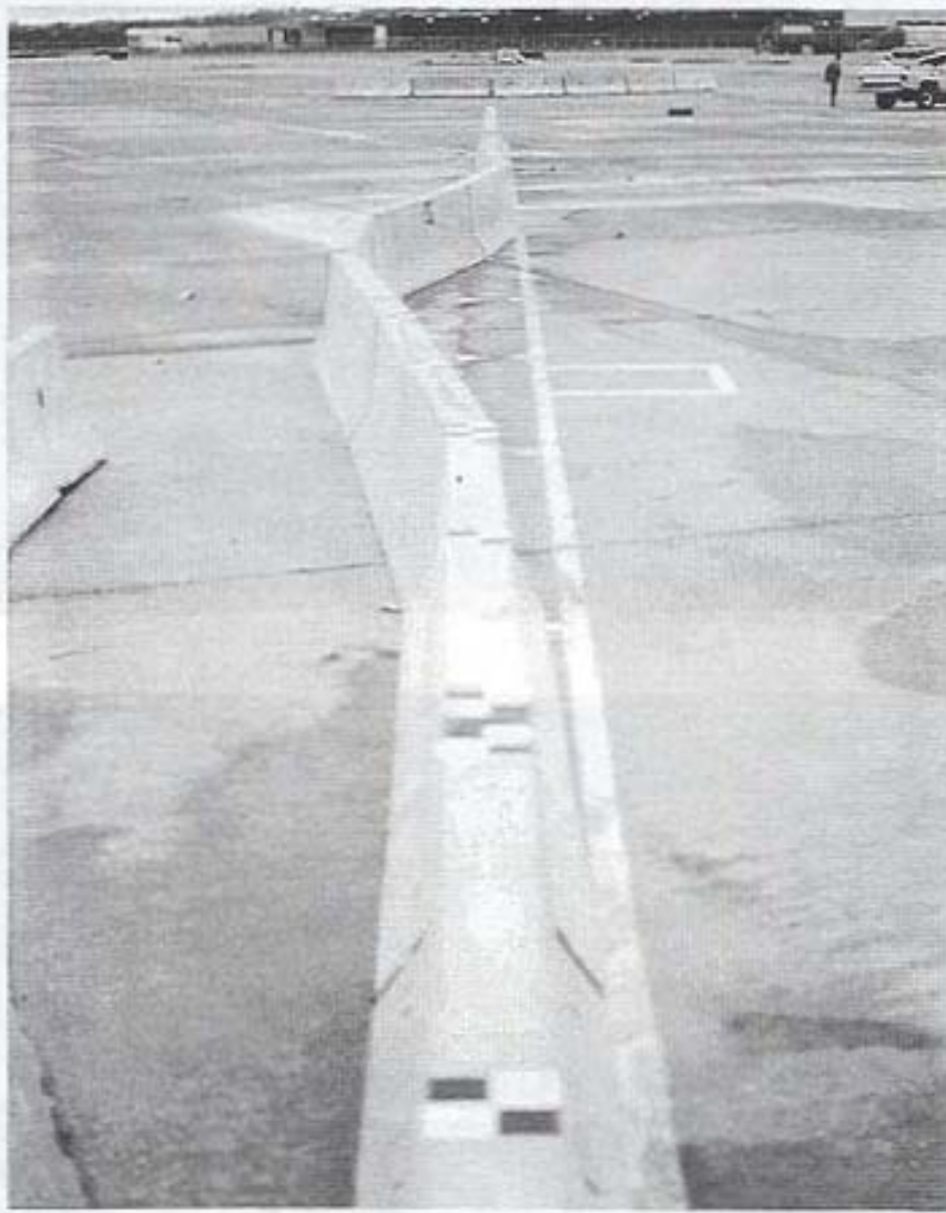
Figure 32. Barrier Damage, Test ITMP-2
