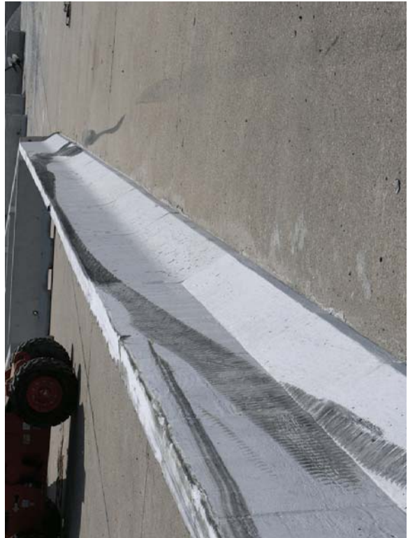
Figure 20. Permanent New Jersey Safety Shape Barrier Damage, Test 2214NJ-2
