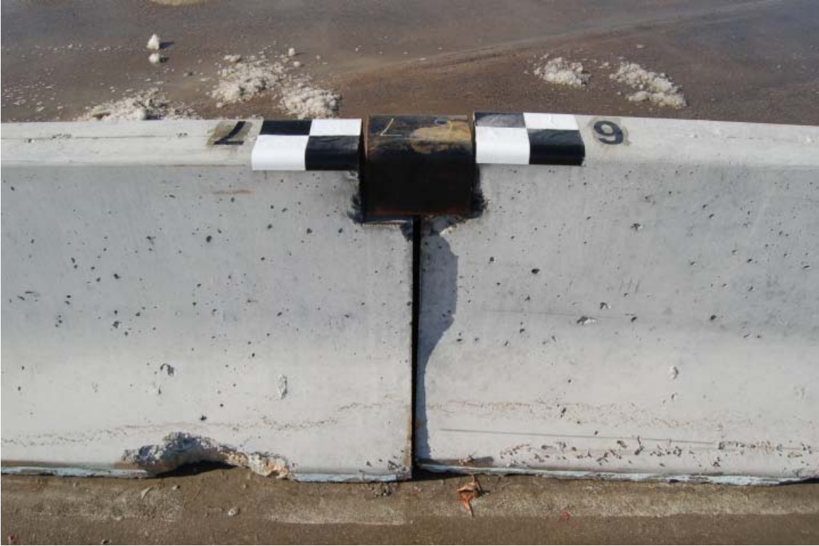
Figure 33. Joint 6-7 Connection Damage, Test NYTCB-4
