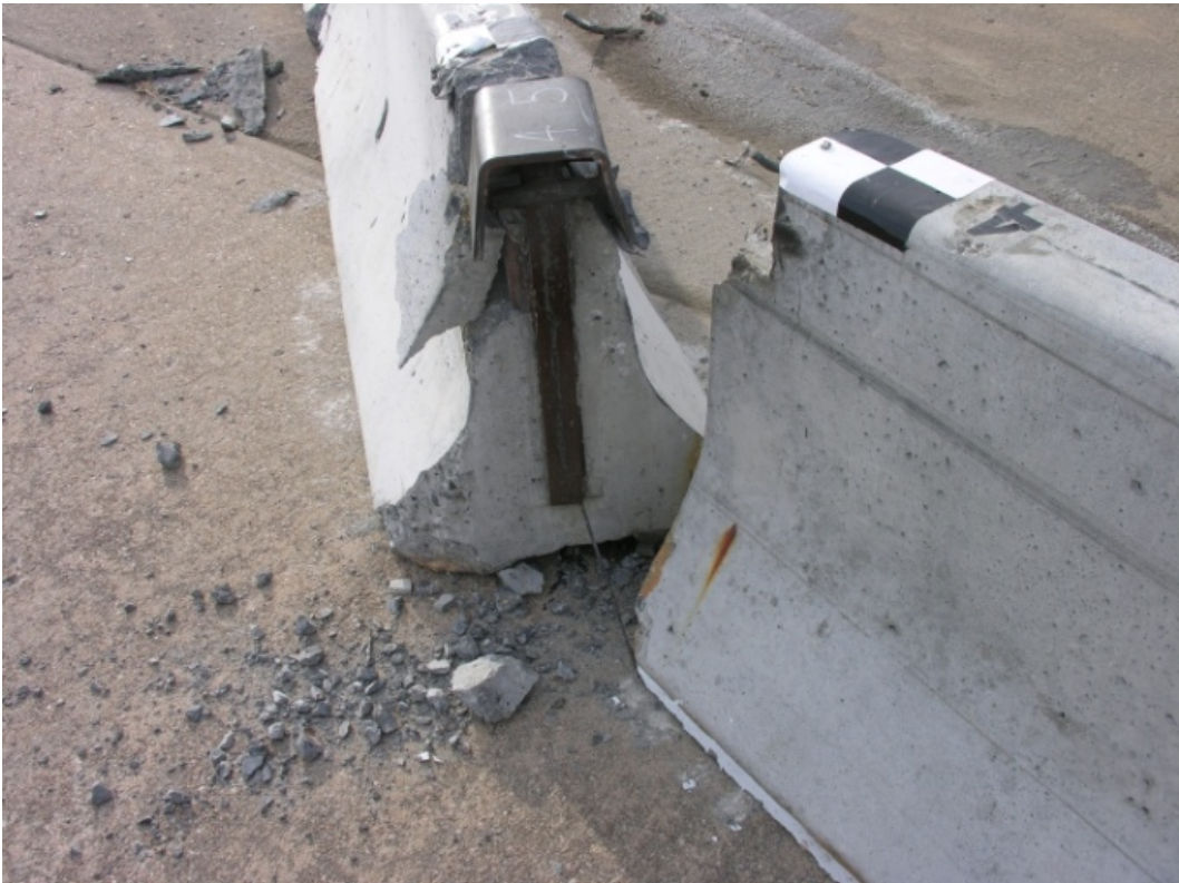
Figure 30. Joint 4-5 Connection Damage, Test NYTCB-4
