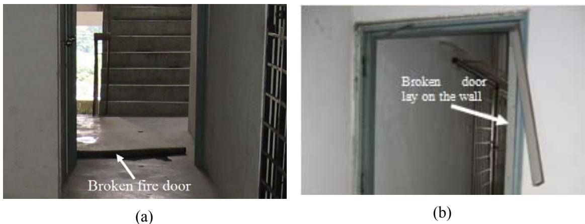
Figure 5.17: (a) Broken fire door lied down on the floor.
