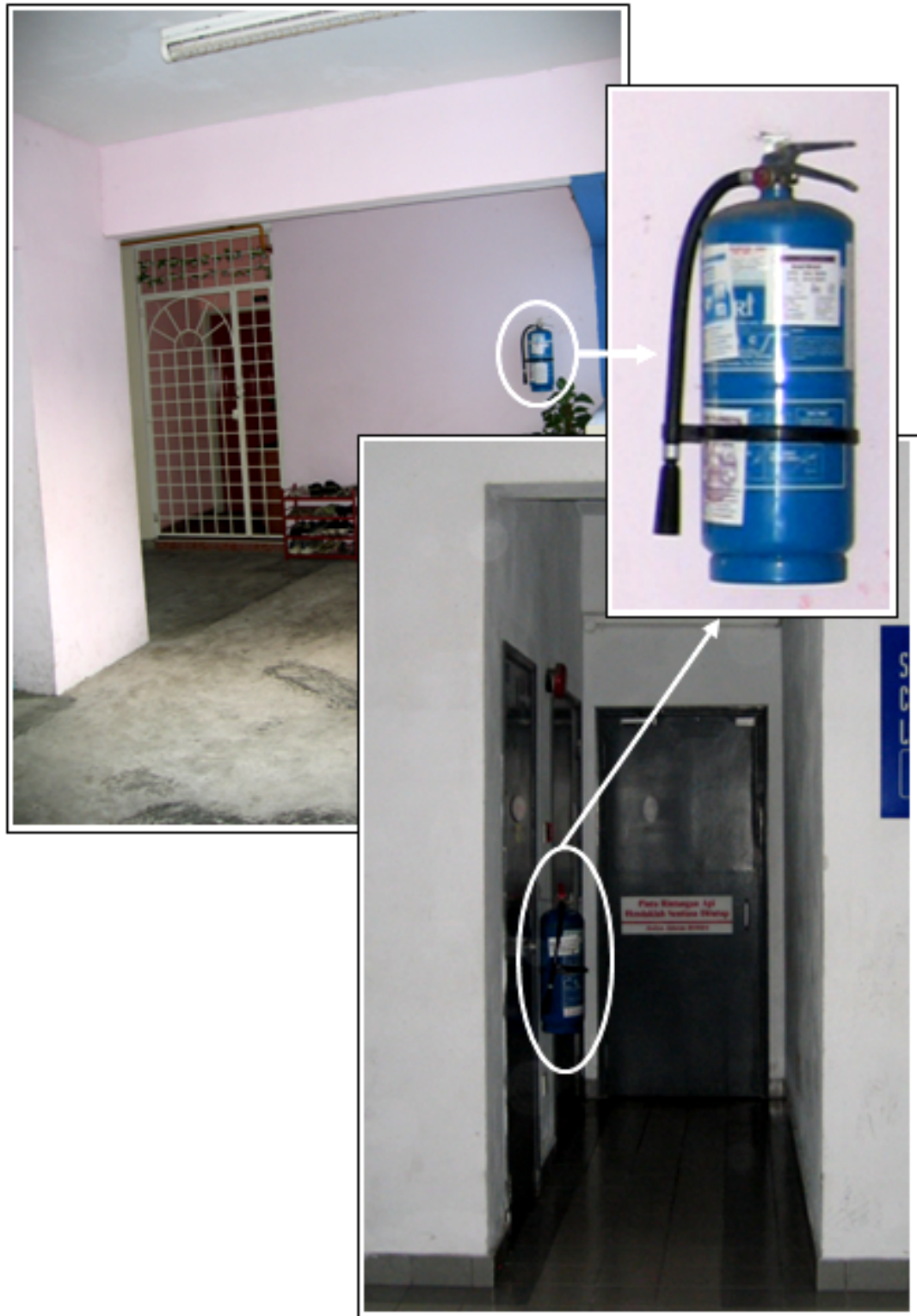
Figure 5.31: Portable fire extinguisher hanging on the wall.
