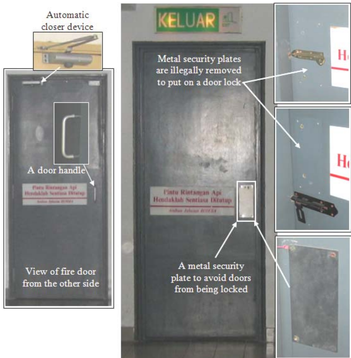
Figure 5.30: Metal security plate from to avoid any locking devices from been fitted on the fire door has been removed by irresponsible person. This vandalism action has jeopardised the safety of others.
