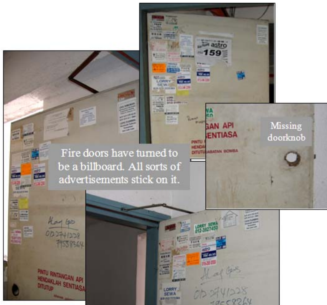
Figure 5.32: Fire doors have been vandalised by sticking all sorts of advertisements on it. Irresponsible persons have turned the fire doors to be a free advertisement billboard.
