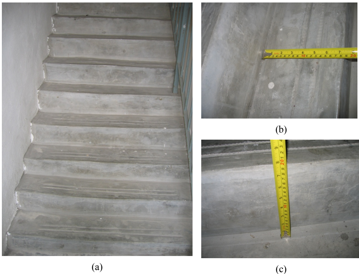
Figure 5.2: (a) Staircase view; tread and riser dimension is about the same size. (b) Tread dimension is only about 7 feet (185mm), whilst minimum requirement is 225mm at least. (c) Riser dimension is about 200mm, whilst maximum dimension should not exceed 180mm.
