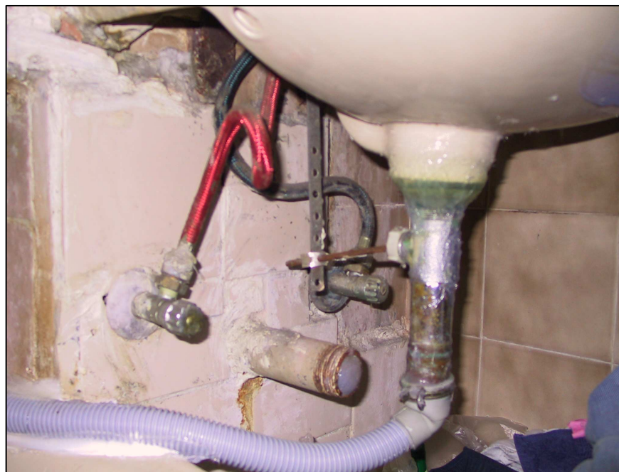
Figure 2.14 Unapproved system adaptation including completely removing the water trap seal provided an open path for cross-contamination (image supplied courtesy of M. Y. Chan, Hong Kong Polytechnic University)
