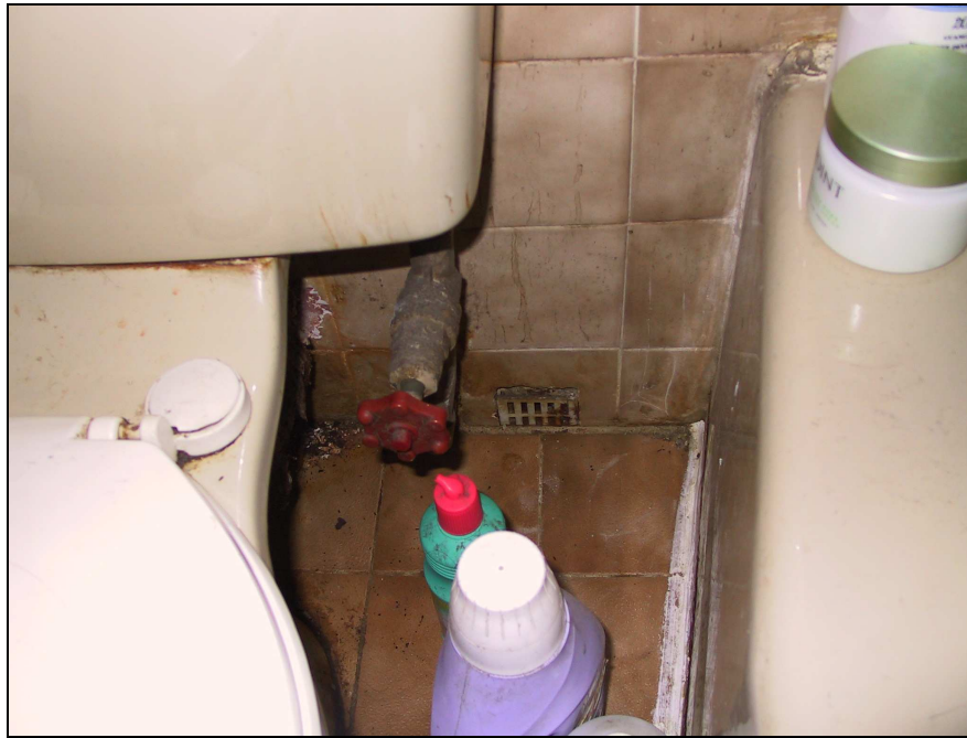
Figure 2.13 Evaporation of the bathroom floor drain water seal provided an open path for cross-contamination (image supplied courtesy of M. Y. Chan, Hong Kong Polytechnic University)
