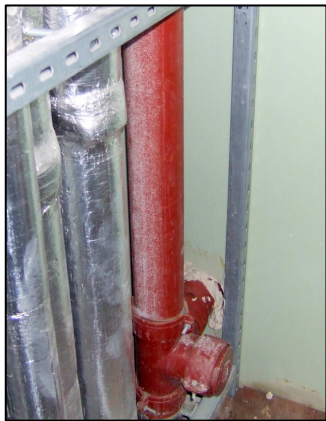
wc branch connection into stack
