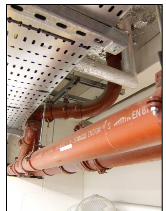
Stack connection to drain pipe at high level in basement
