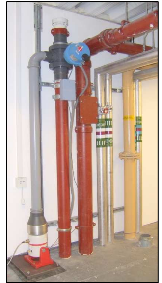
Transient entry device installed on Stack 3
