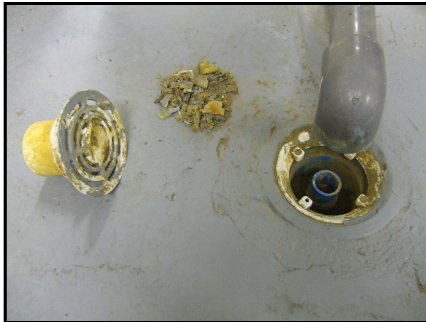
Figure 5.33 The boiler room floor gully was found to be completely dry and was filled with debris
