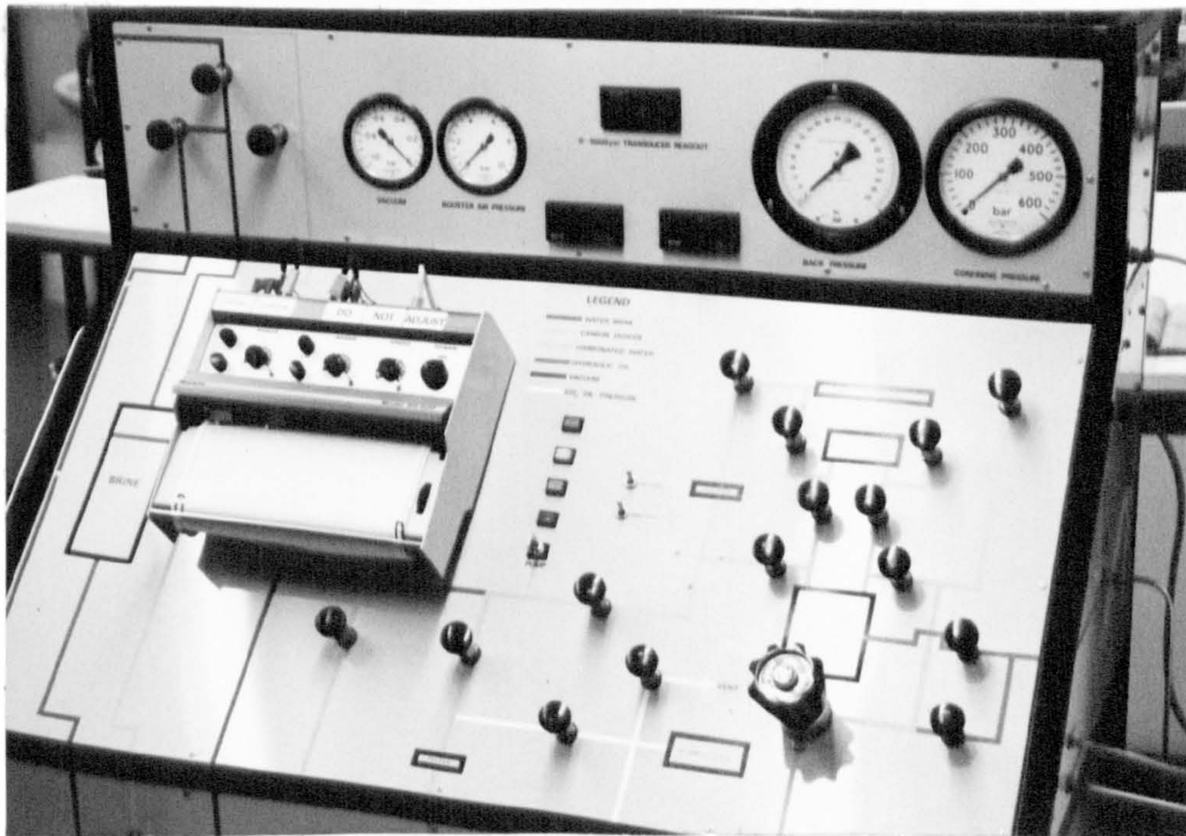
PLATE II-2. CLOSE-UP OF CONTROL PANEL
