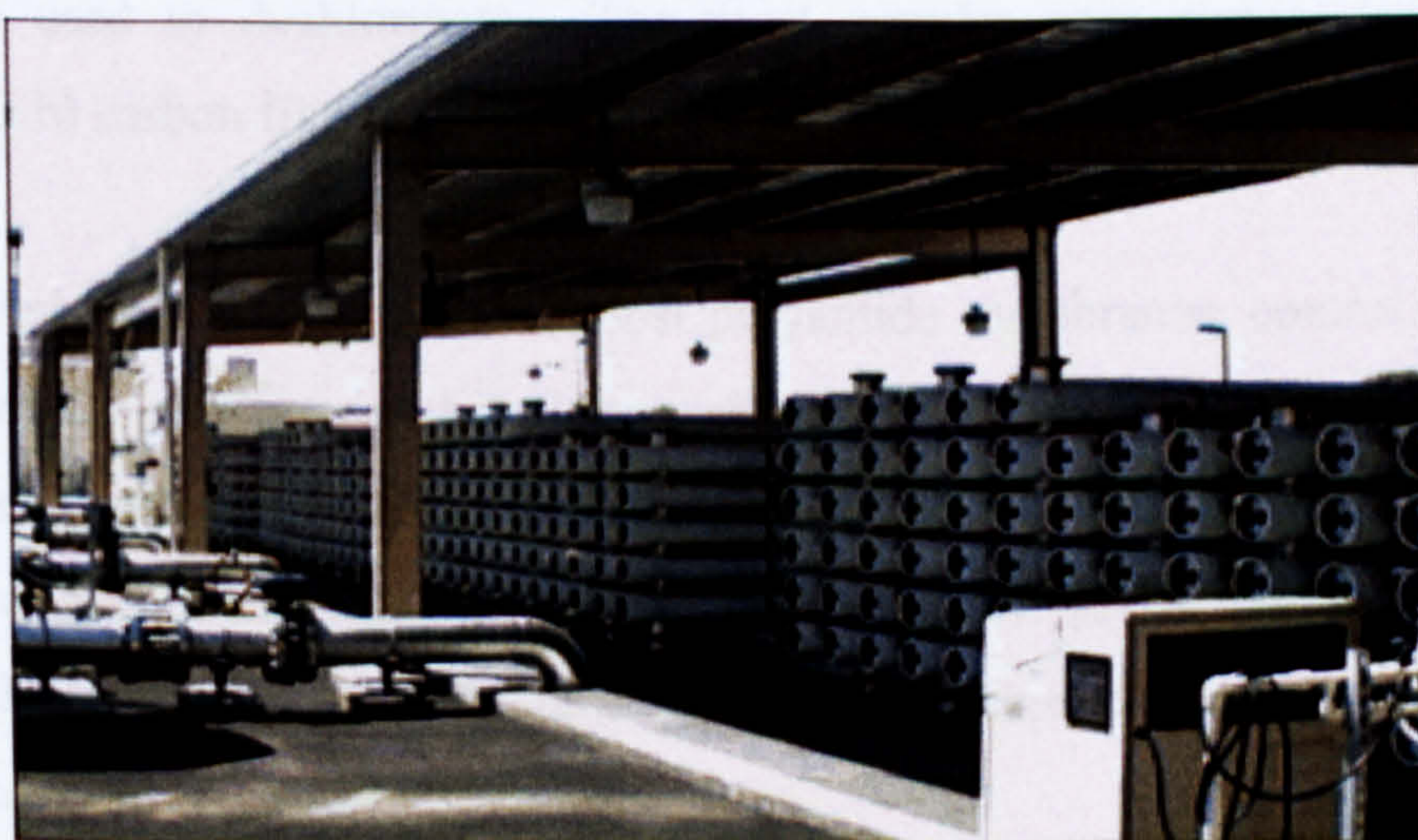
ESPA installation, 5 MGD, in Carson, California
