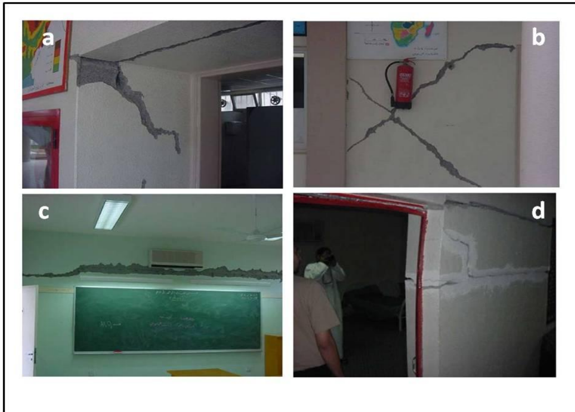
Figure 44: The impact of earthquake Masafi 2002 on the buildings of Masafi, Picture (a) and (b) shows the effects of the earthquake on the walls of Masafi schools, picture (c) shows a crack the top board in a classroom, picture (d) shows the big crack in Masafi house. (AUS 2008).
