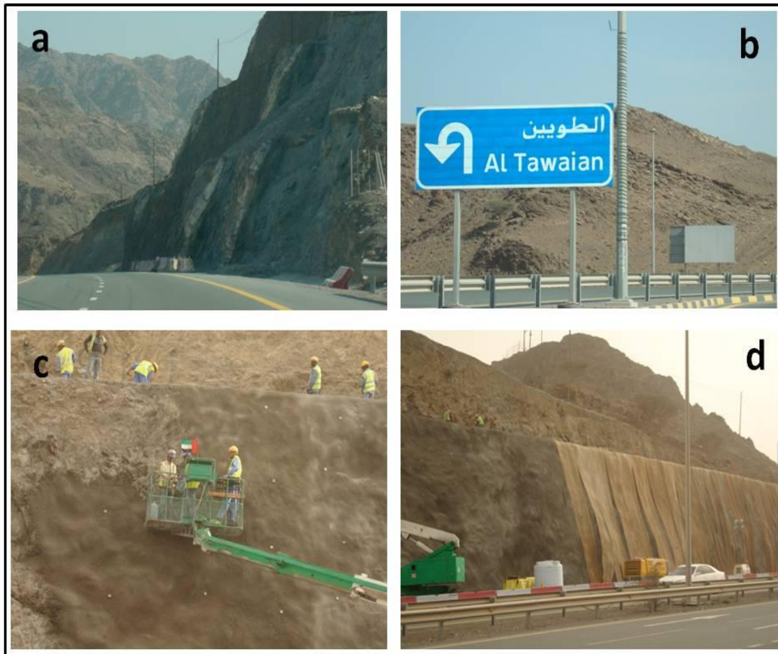
Figure 50: Tawaian-Dibba Road and response stage. Picture (a) Tawaian-Dibba Road, (b) Tawaian Road, (c) The road maintenance operation (d) One of the stages of the maintenance of the road.
