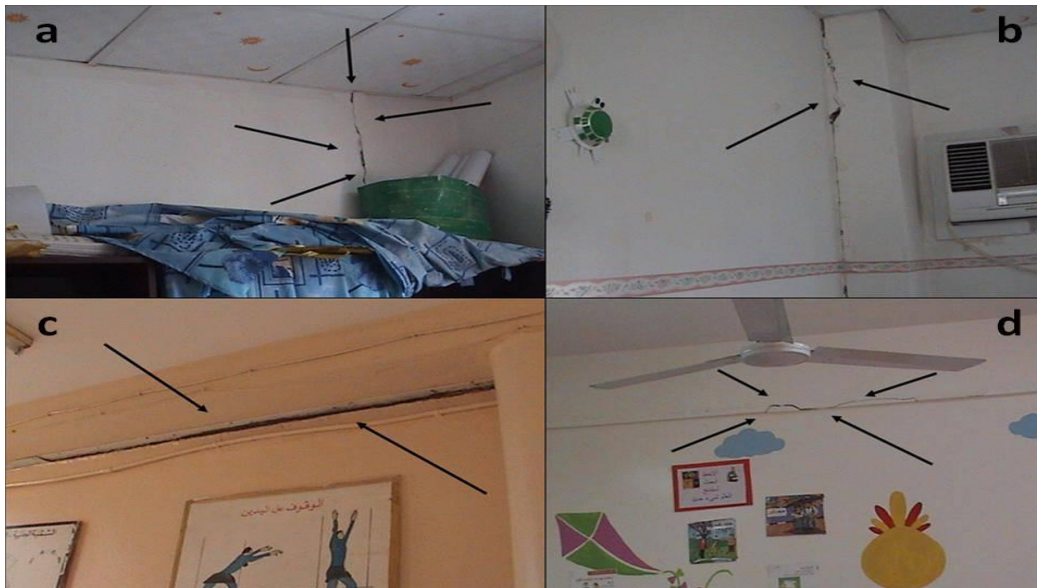
Figure 67: The effects of earthquake on Rumaitha School, pictures (a, b, c, d) shows effects in classroom.
