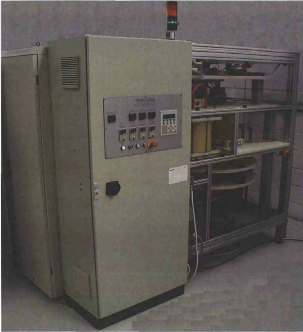
Figure 65 - Completed industrial PFM, showing operator station, mechanical handling control cabinet (front) and high voltage cabinet (left rear)
