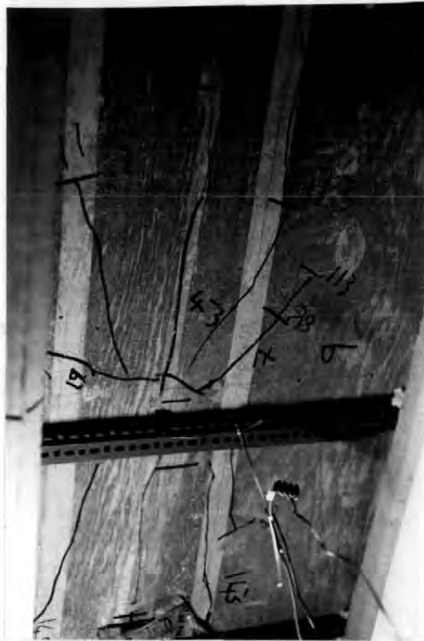
Figure 8.24: Crack pattern under single wheel
