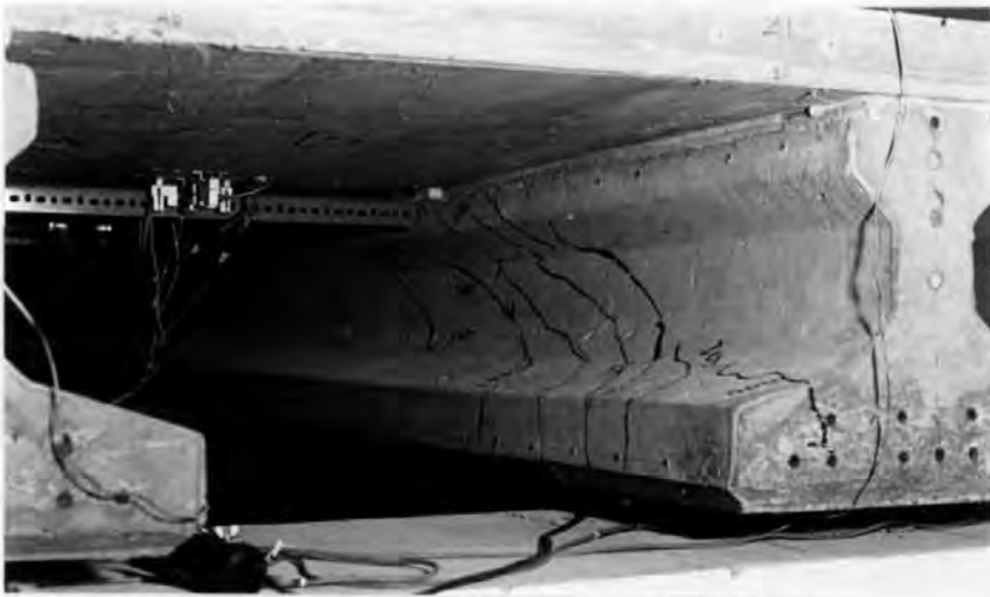
Figure 8.16: Shear cracks in Beam B
