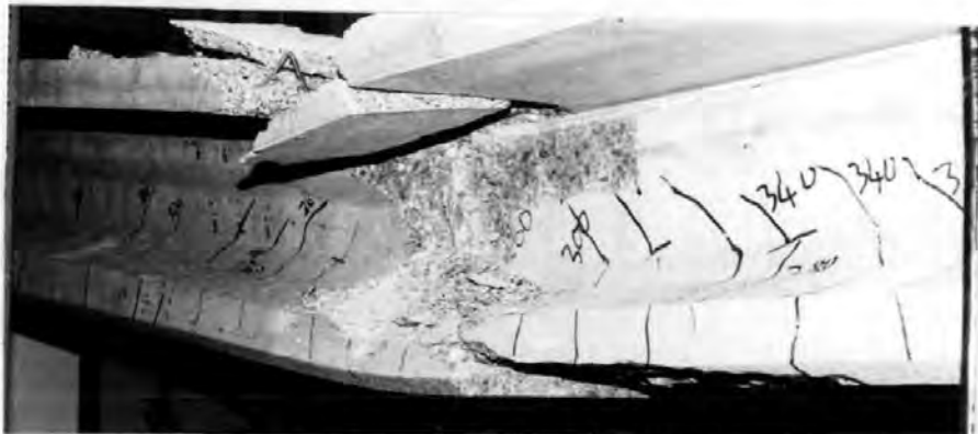
Figure 8.39: Beam after failure
