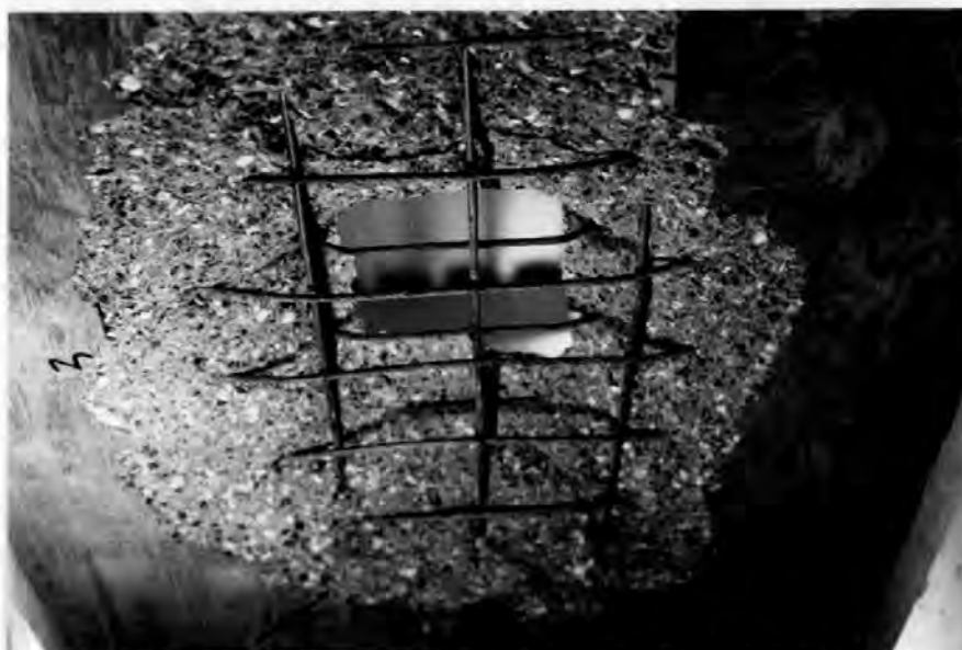
Figure 8.25: Failure cone viewed from below
