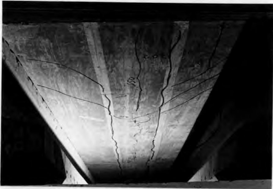
Figure 8.17: Soffit cracks under wheel 4
