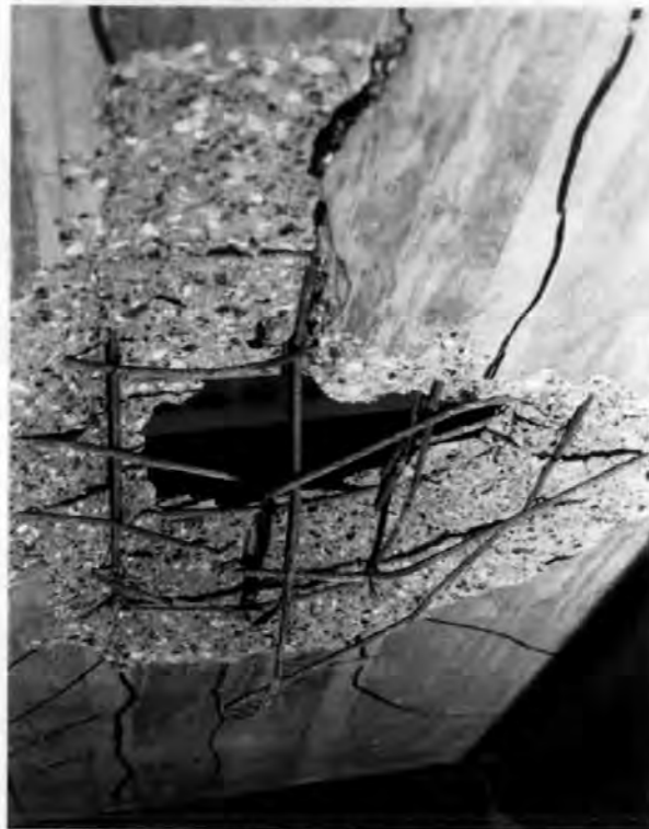
Figure 8.21: Failure cone viewed from below
