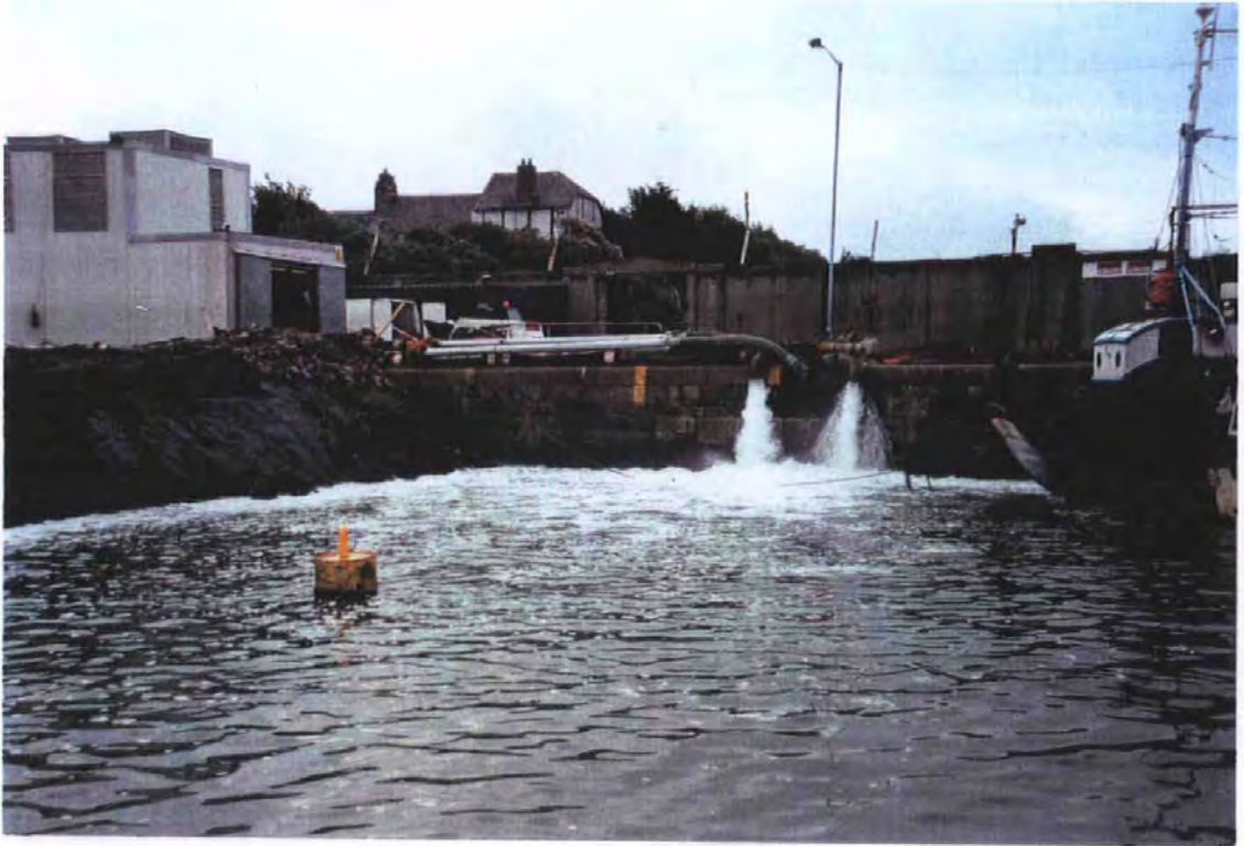
Plate 1.3. View to the south in the eastern arm of the harbour showing the clay-cored coffer dam (left) and the extensive pumping of water from behind the coffer dam into the main harbour to maintain the dry dock.
