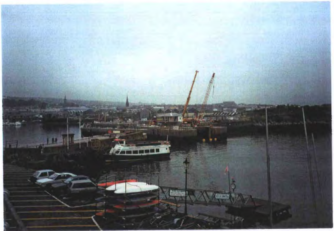
Plate 1.4. View to the north east overlooking the harbour mouth with the lock chamber (centre) in its final position. The control room can be seen and the scheme is in the final stages of completion. Note the restricted temporary harbour entrance (behind vessel) before the removable stop-log gate was positioned.
