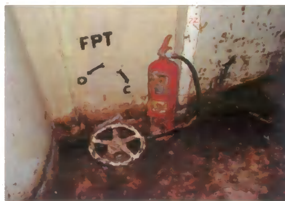
Fig.5.15 Damaged portable fire extinguisher
