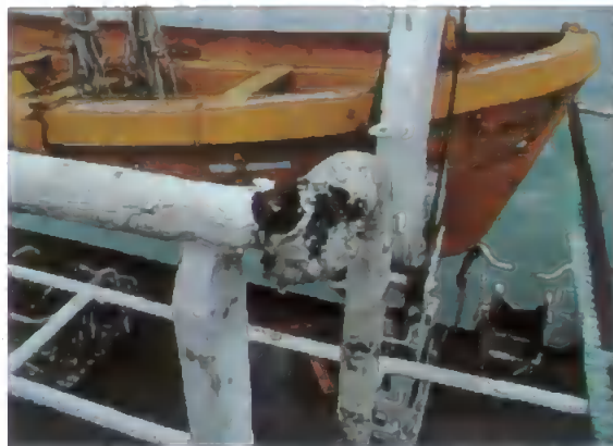
Fig. 5.12 Broken life boat davit
