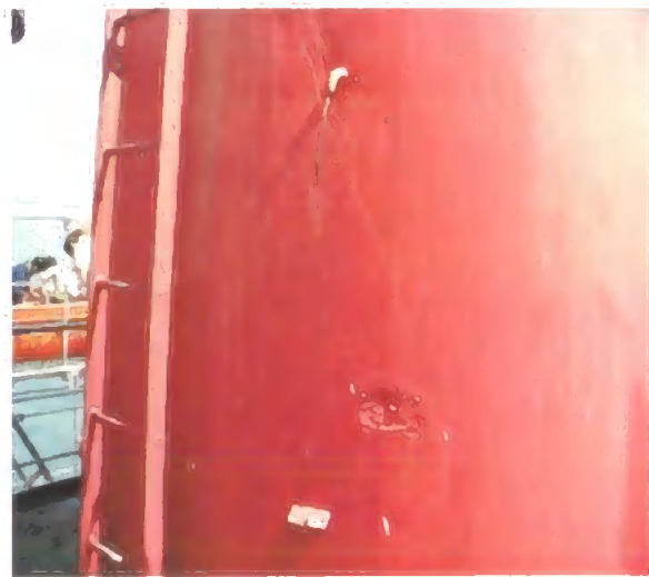
Fig. 5.8 Broken closing wire for vent flap
