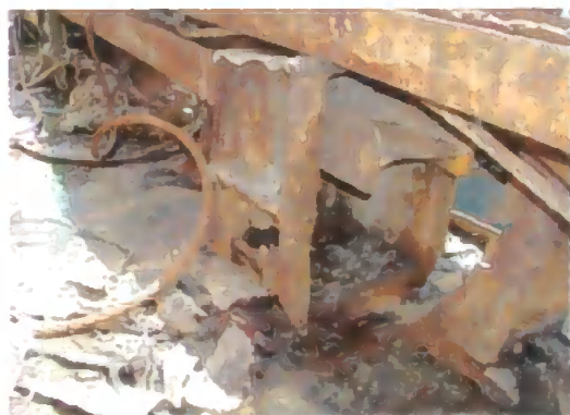
Fig. 5.1 Corroded stanchion on deck
