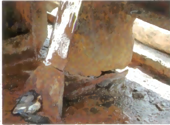
Fig. 5.3 Cracked stiffener on deck
