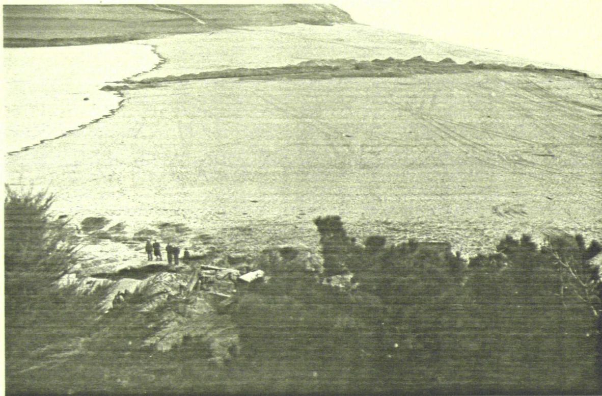
Plate 3.14: Mechanical excavators being used to clear the adit entrance of shingle, February 1979.
