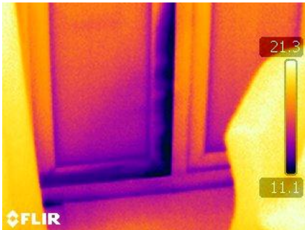
Figure 6.3: Example thermal image showing dark (cold) areas where there is cold air ingress around the surround of the doorway.
