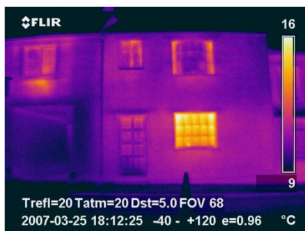
Figure 4.1: Example of thermal image showing the brighter area, single glazed window.
