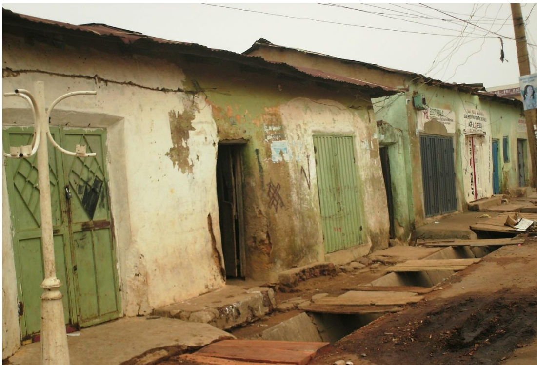
Figure 4.16: The effect of electrical installation and government services (road, drainage, etc.) on adobe buildings
