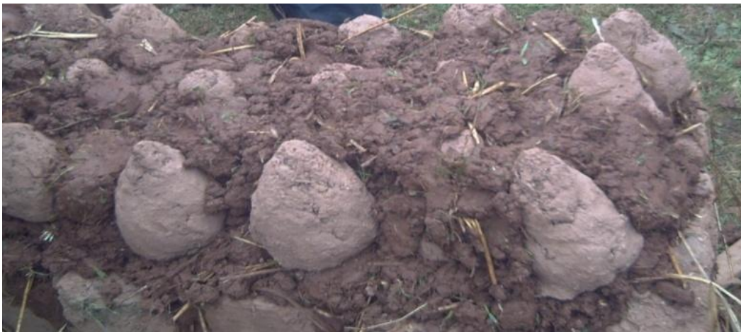
Figure 5.11: Demonstration tubali wall under construction during the 'Cob Week' at the University of Plymouth
