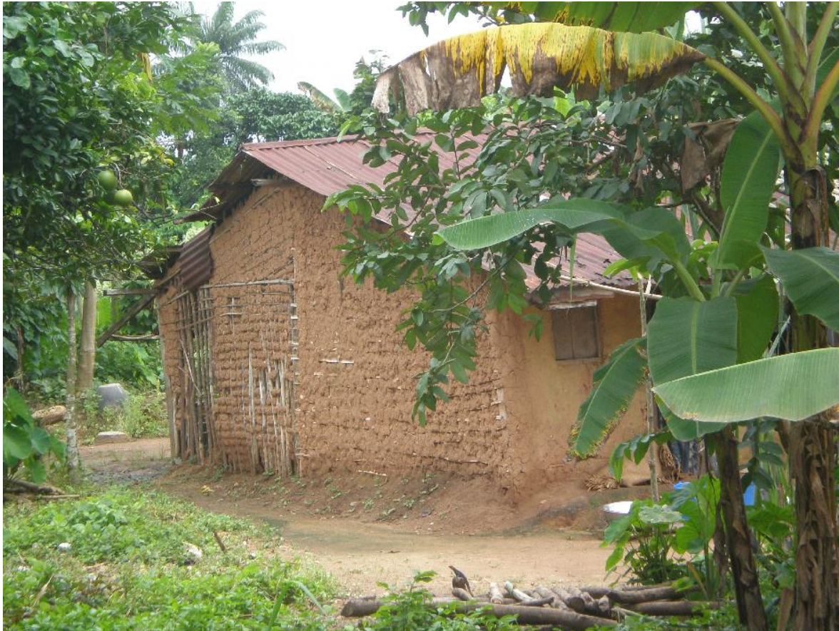
Figure 5.34: An eroded wattle and daub
