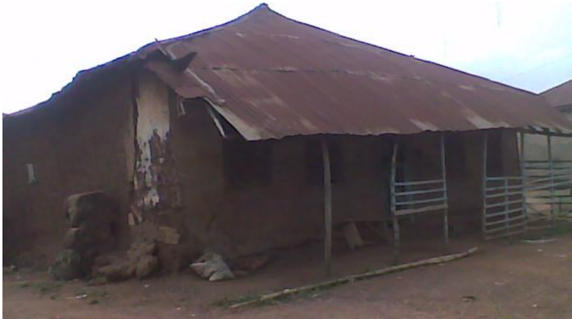
Figure 5.30: A cob building with vertical crack
