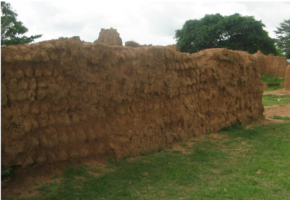
Figure 5.12: A ruined tubali wall in Zaria City
