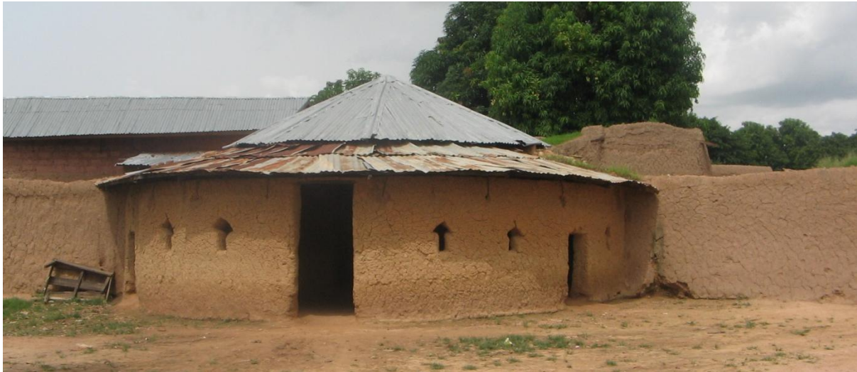
Figure 5.19: Circular plan adobe building with conical roof made from corrugated iron sheets
