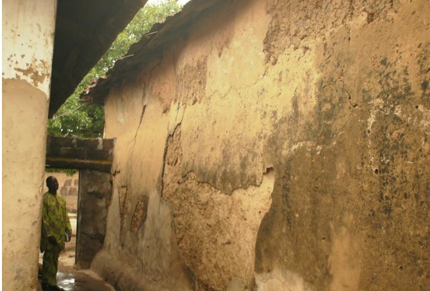
Figure 4.18: Roof of adjoining property affecting adobe wall in another property
