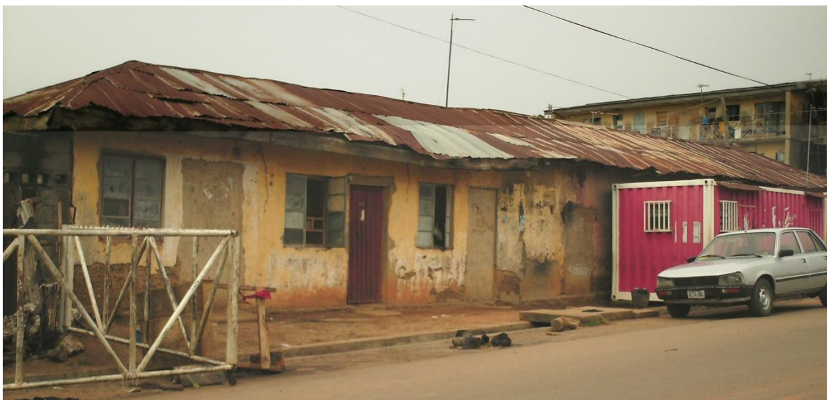
Figure 4.9: Adobe building with sagged roof, replaced roofing sheets, two sealed doors and cement based rendering. Note also the steel container use as part the building extension.
