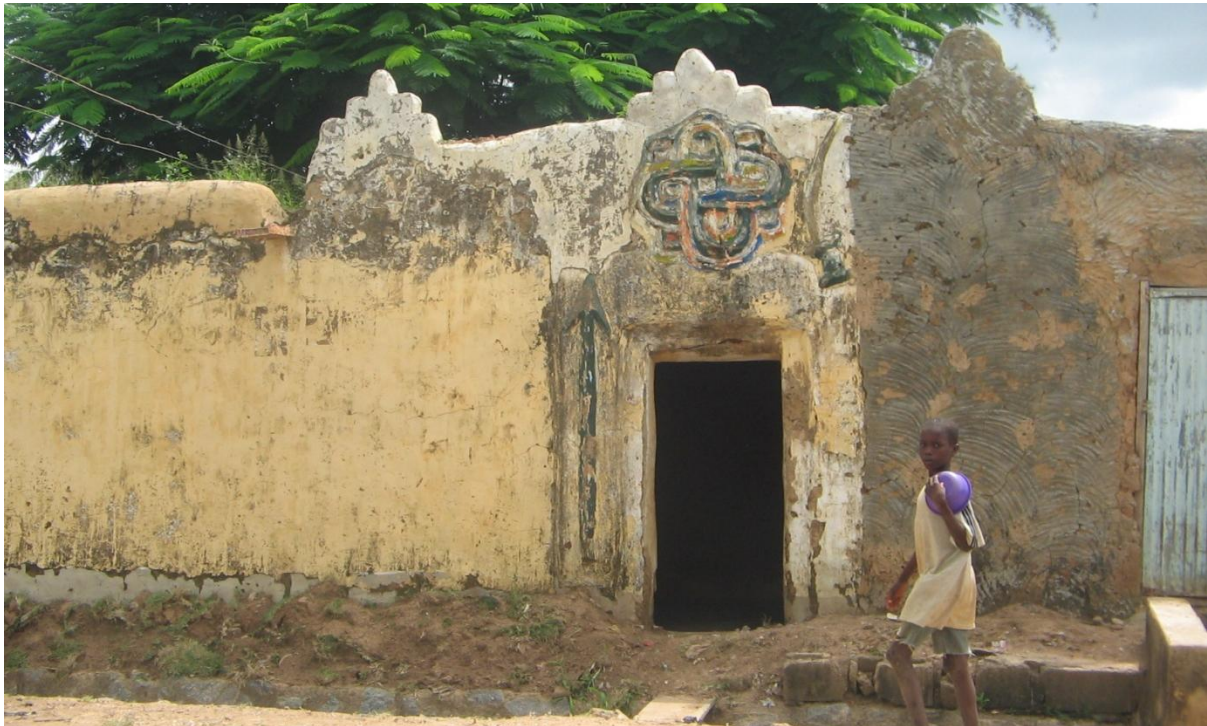
Figure 5.20: A dilapidated adobe building with cementious render
