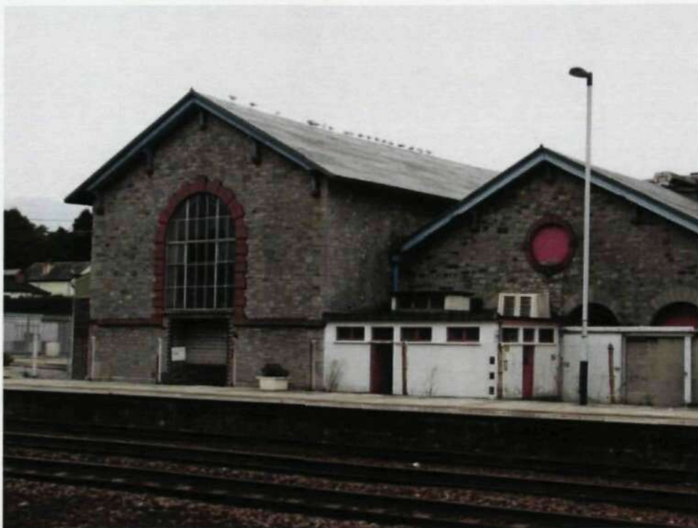
Figure 2.60 Totnes, Devon, one of the surviving Engine Houses of Brunel's Atmospheric Railway.
