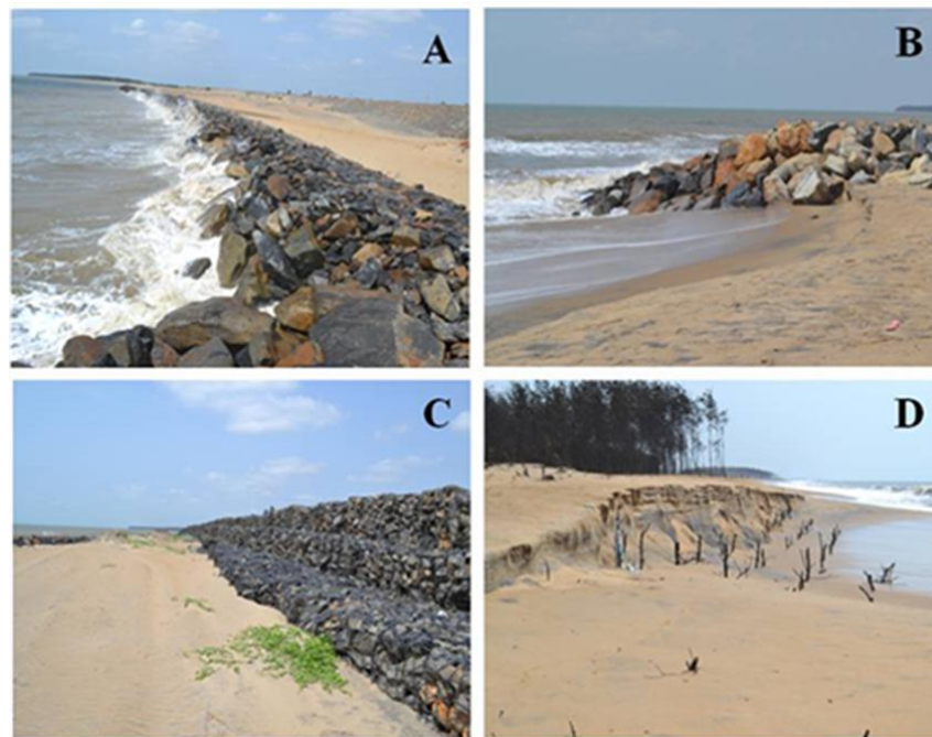
Fig. 4 — Field photo captured at erosion sites near Paradeep Port (A) and near Satavaya beach (B) showing the sea wall constructed to prevent the erosion, the wire mesh rock wall constructed at Pentha coast of Jagatsingpur District (C) and erosion at Mahanadi River mouth (D) reveals the severity of the erosion. Locations of these photos are marked on the map (Fig. 3)
