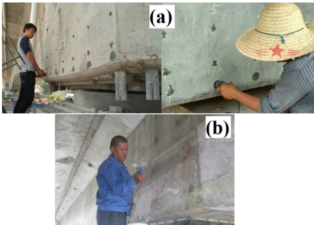
Fig.11 — field test process: (a). Field data acquisition (receive sensor); (b). Field data acquisition (hammering)
