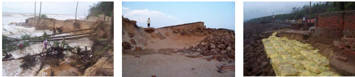
Figure 5. a) The sea erodes deep into the coastal tree cover in Sankarpur b) The sea wall that was once built has been broken by the waves at Old Digha c) The concrete path that connects Digha to old Digha has been broken by the waves is being temporarily repaired.
