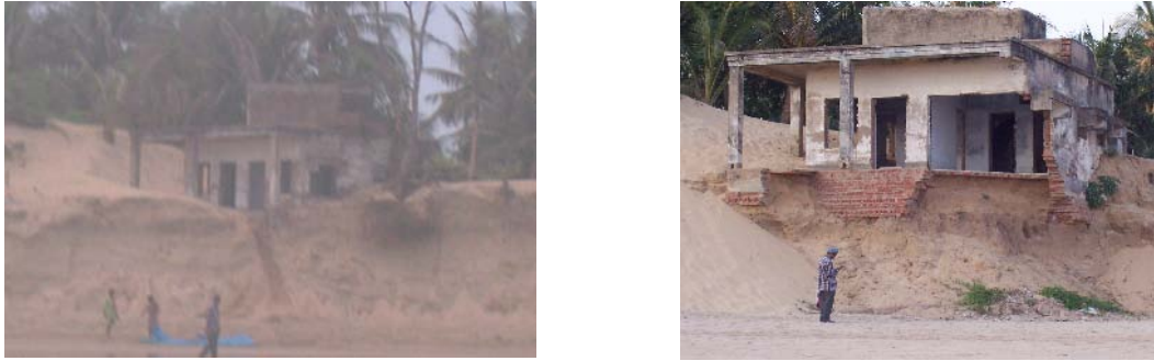
Fig. 4— a) A house on Sankarpur beach in 2004 and 2005. b) In 2006, the house was swallowed by the sea
