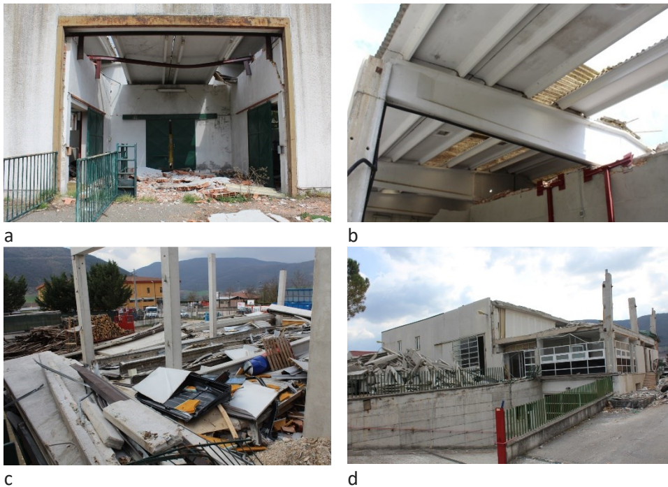
Figure 2.4 Absence of mechanical devices among structural elements: Partial a) e b) and complete c) e d) collapses of roof elements.
