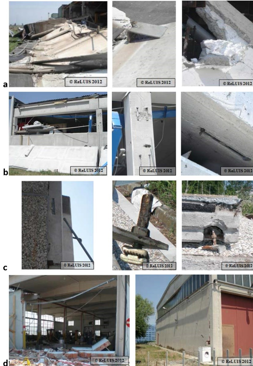
Figure 2.3 Damage of a) vertical and b), c) horizontal cladding panels and d) infill masonry observed during 2012 Emilia Romagna seismic event.
