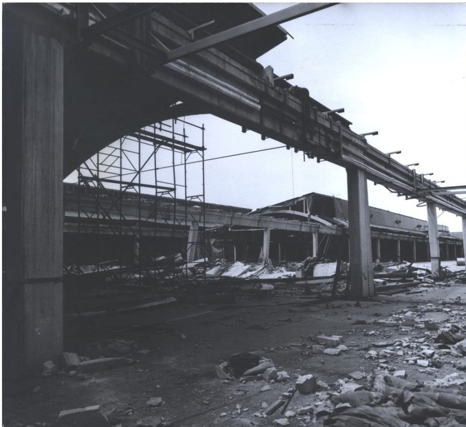
Figure 2.2 Historical photos concerning the damages suffered by the industrial company during the 1976 Friuli earthquakes https://www.snaidero.it/gallery-40°-anniversario-terremoto-friuli .
