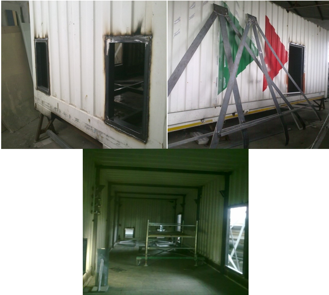
Fig. 5.7: Modification's phase of the containers – Mobile plant, HydroWEEE demo
