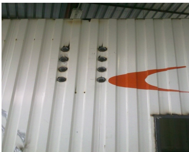
Fig. 5.8: Opening for piping – Mobile plant, HydroWEEE demo
