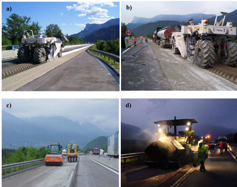
Figure 6. 7 Photos taken during the construction of the experimental pavement section: a) First recycler pass for mixing RA with RAG; b) Subbase stabilization with bitumen emulsion; c) Subbase compaction by means of pneumatic tire roller; d) Laydown of the HMA base layer.
