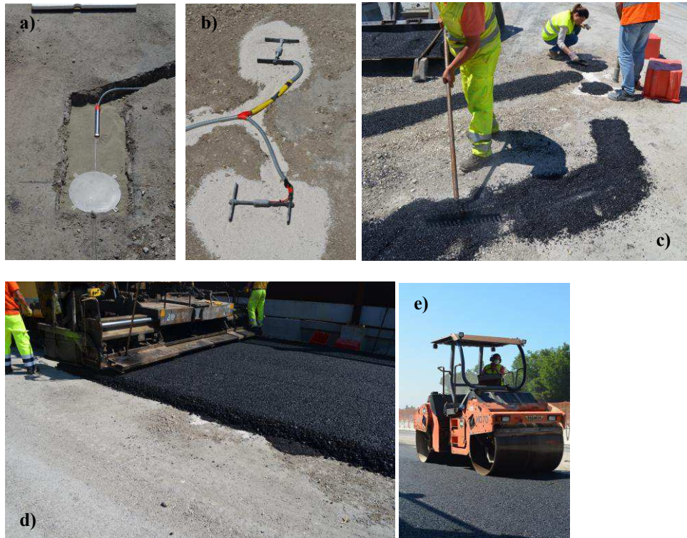
Figure 8. 9 Second part of instruments installation: a) placing of EPC3; b) installation of ASG1 and ASG2; c) filling and leveling with 8 mm-sieved asphalt concrete in order to protect ASGs; d) HMA layers laydown and e) final compaction.
