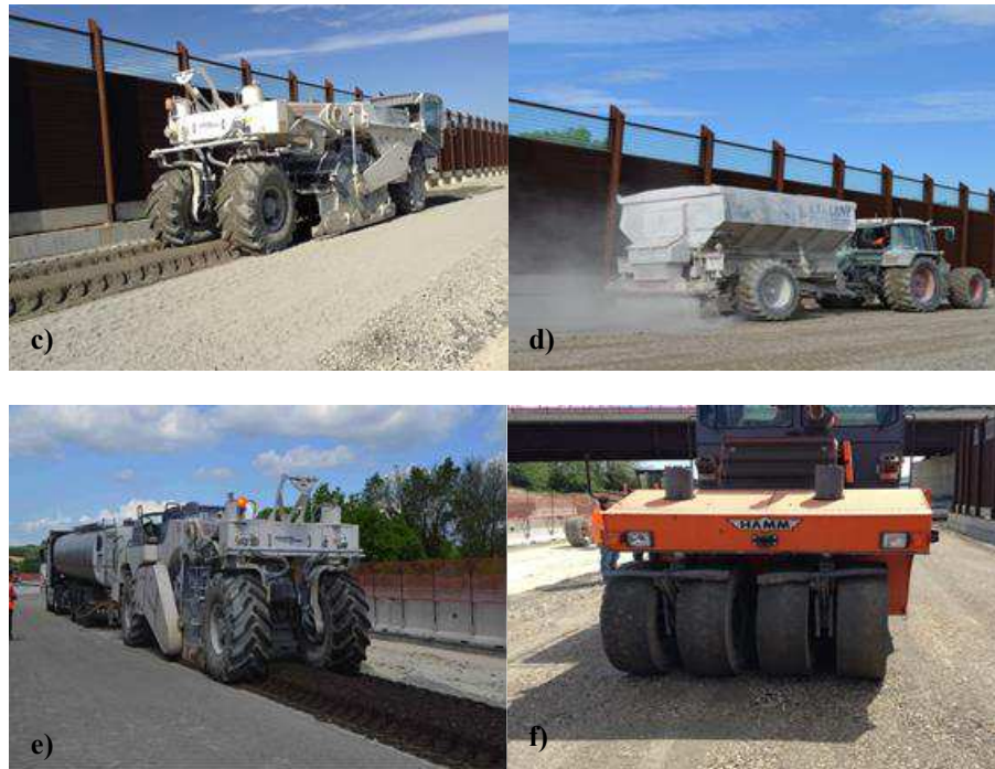
Figure 8. 7 Construction of CBTM and CTM layers: a) RA material restoring; b) placing of RAg layer; c) mixing of the milled material; d) spreading of cement; e) stabilization with bitumen emulsion and f) final compaction.
