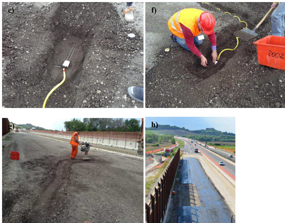
Figure 8. 8 First part of instruments installation: a) placing of EPCs; b) covering with protective material (clean sand and 4 mm-sieved subbase material); c) Placing of cables protected using a flexible steel conduit; d) cavity preparation for TDR and temperature probes; e) placing of TDR and temperature probes; f) Protection of TDR and temperature probes with 4 mm-sieved subbase material; g) trench compaction by portable Marshall hammer; h) partial application of emulsion tack coat.
