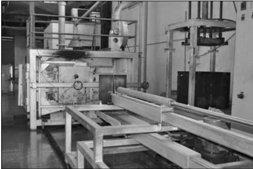
Fig 1: Pilot Coke Oven facility at JSW R&D and SS Centre
